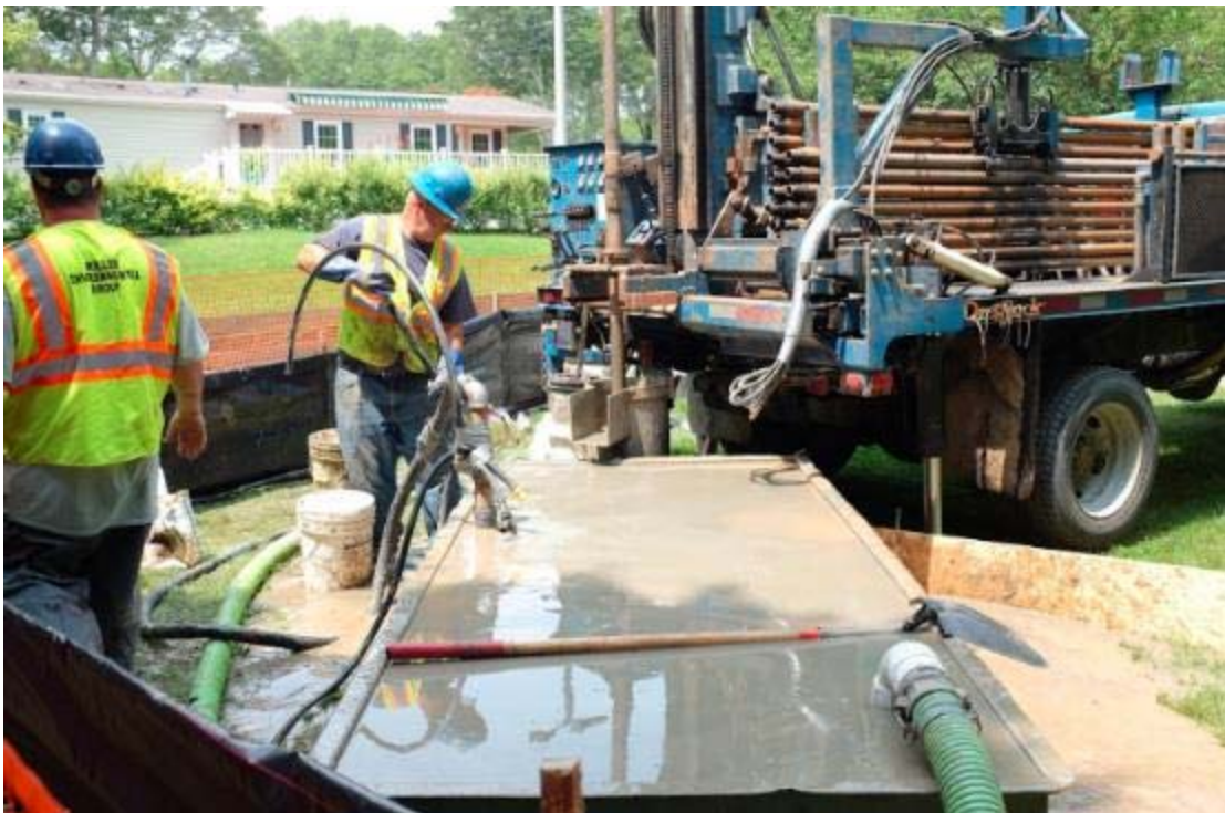
Photo of the well cuttings being shoveled out of the portable mud pit at the Glenwood Village Site.
