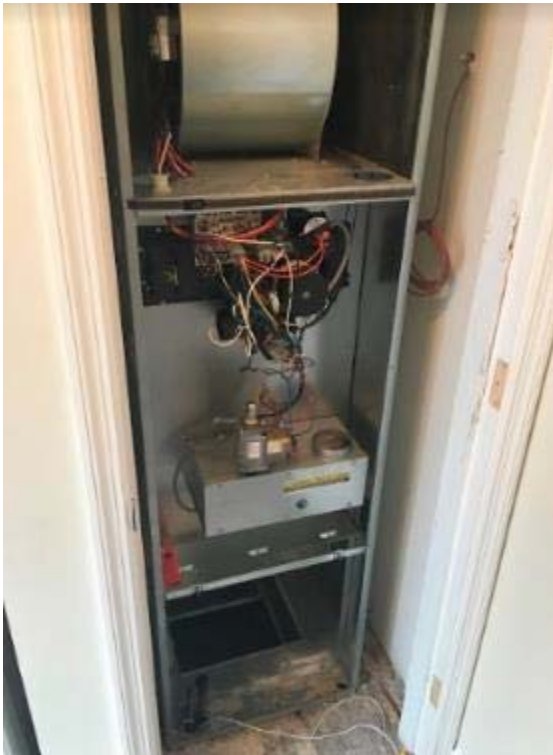
The indoor split system with front panels removed at the Glenwood Village Site.
