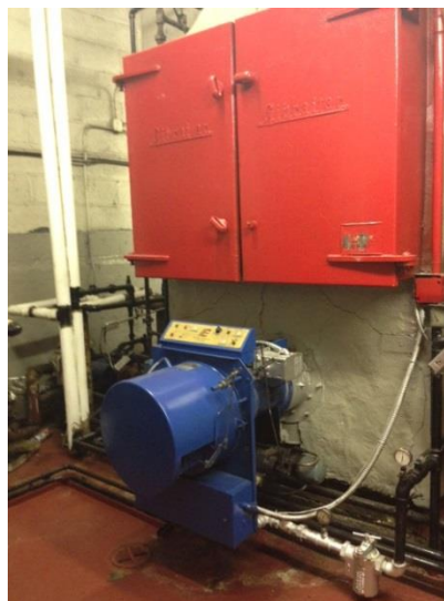
Fig 4.1.1: Current Boiler in the Building
