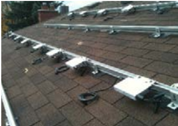
A Solar Electric Racking System
