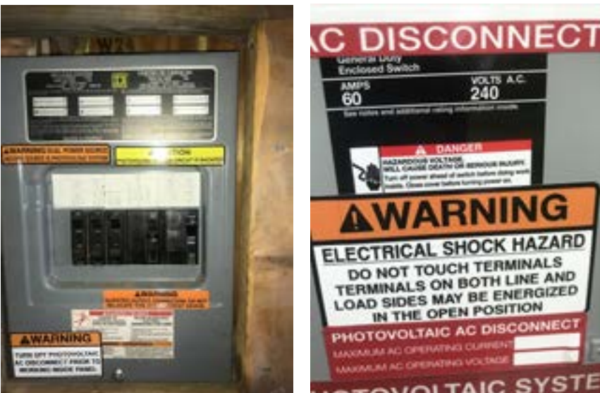
Photo 11: AC disconnect/load center manufacturer's label obscured: NEC 110.21
