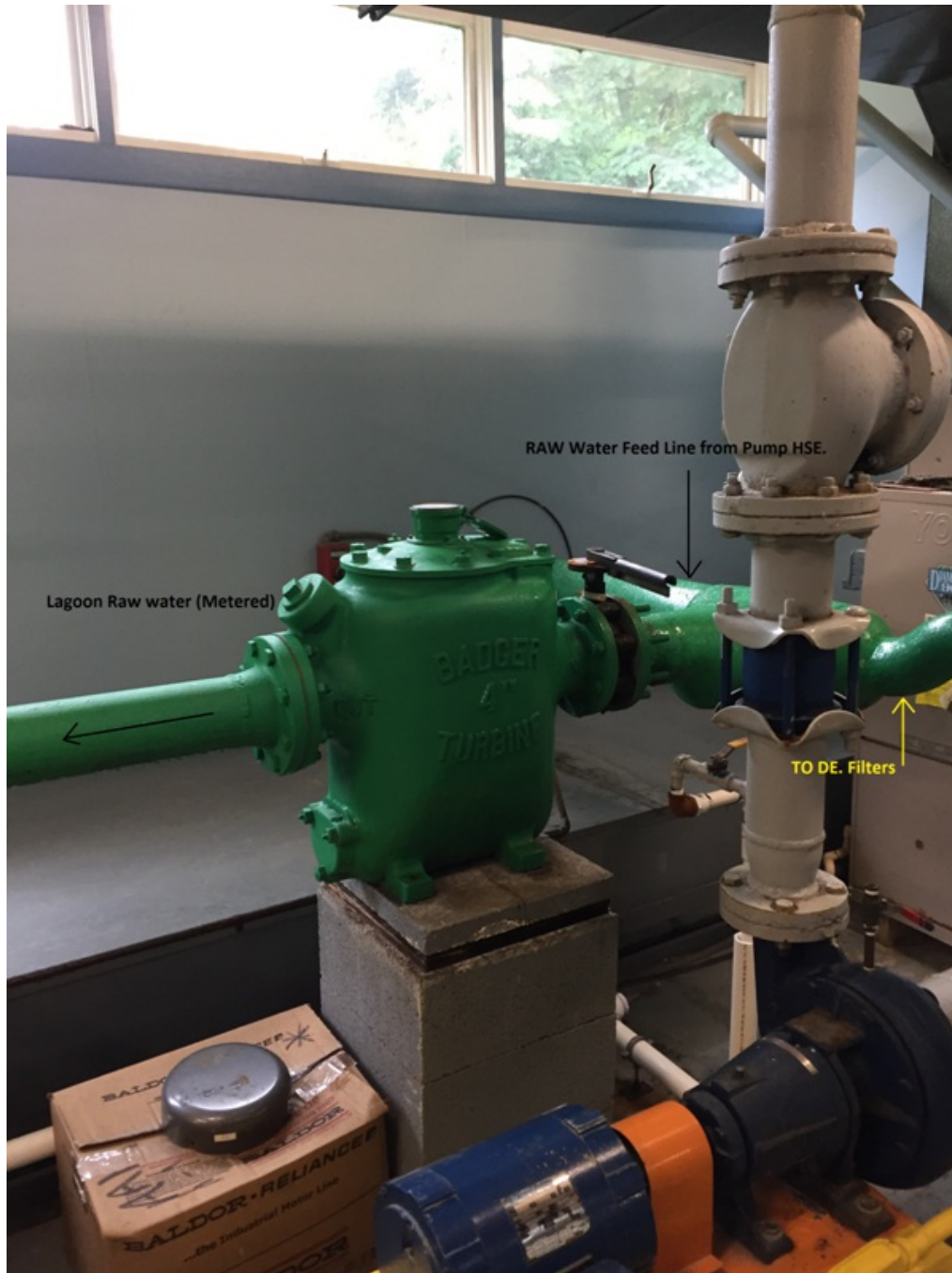
Lagoon meter located in water treatment plant
