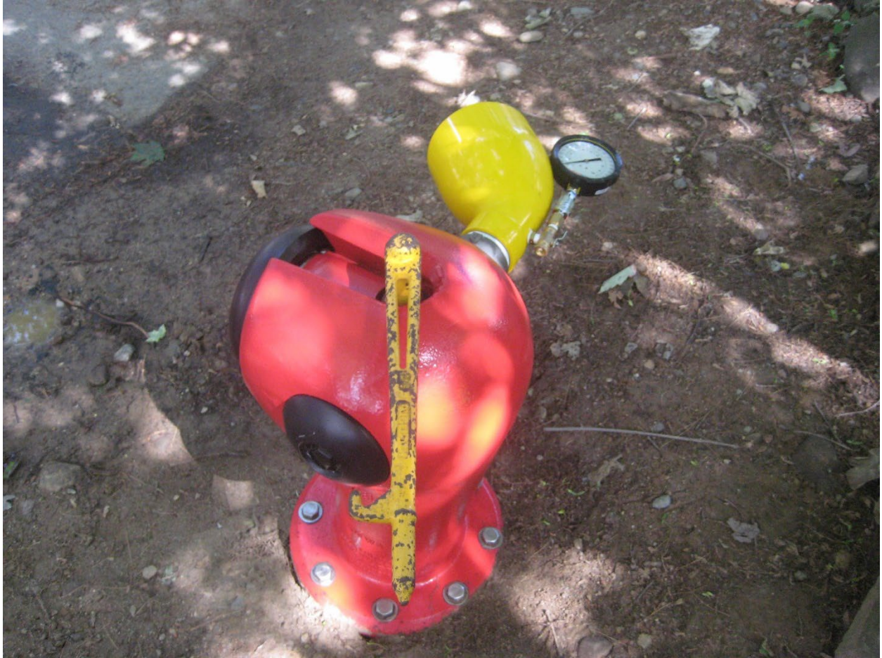
Hydrant 1-119 – Hydrant with diffuser – June 10, 2021
