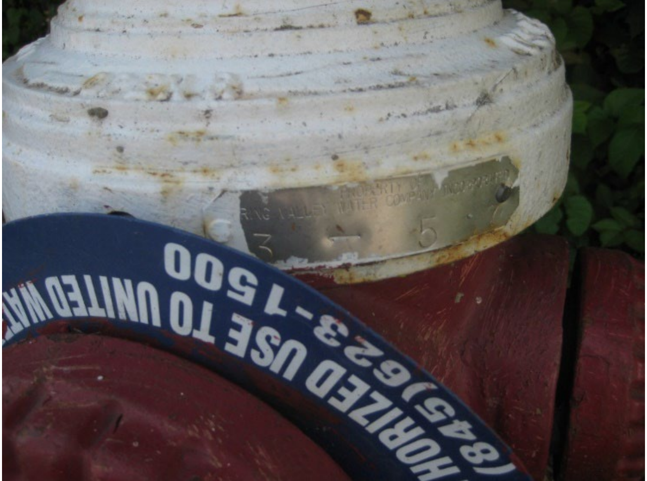
Hydrant 3-5 Nameplate which indicates the hydrant number – June 10, 2021
