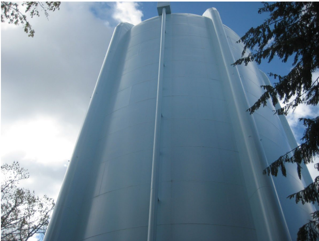
Photo 2 – SUEZ Spring Valley Standpipe – April 30, 2021
