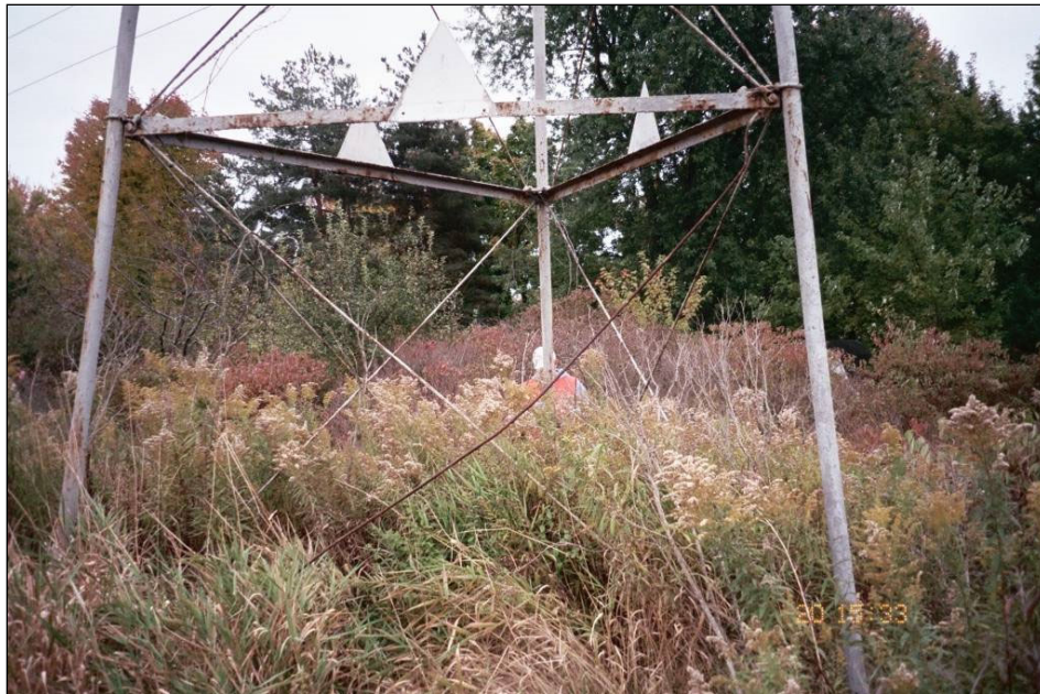
FIGURE E-4.2-1 BENT AND BROKEN BRACINGS
