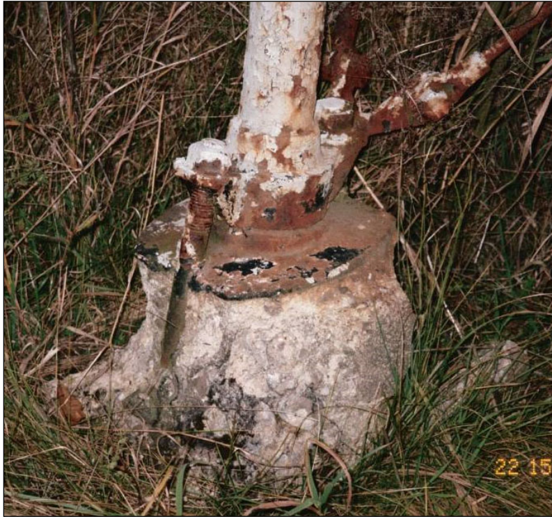
FIGURE E-4.2-2 SPALLED CONCRETE AND EXPOSED ANCHOR BOLTS
