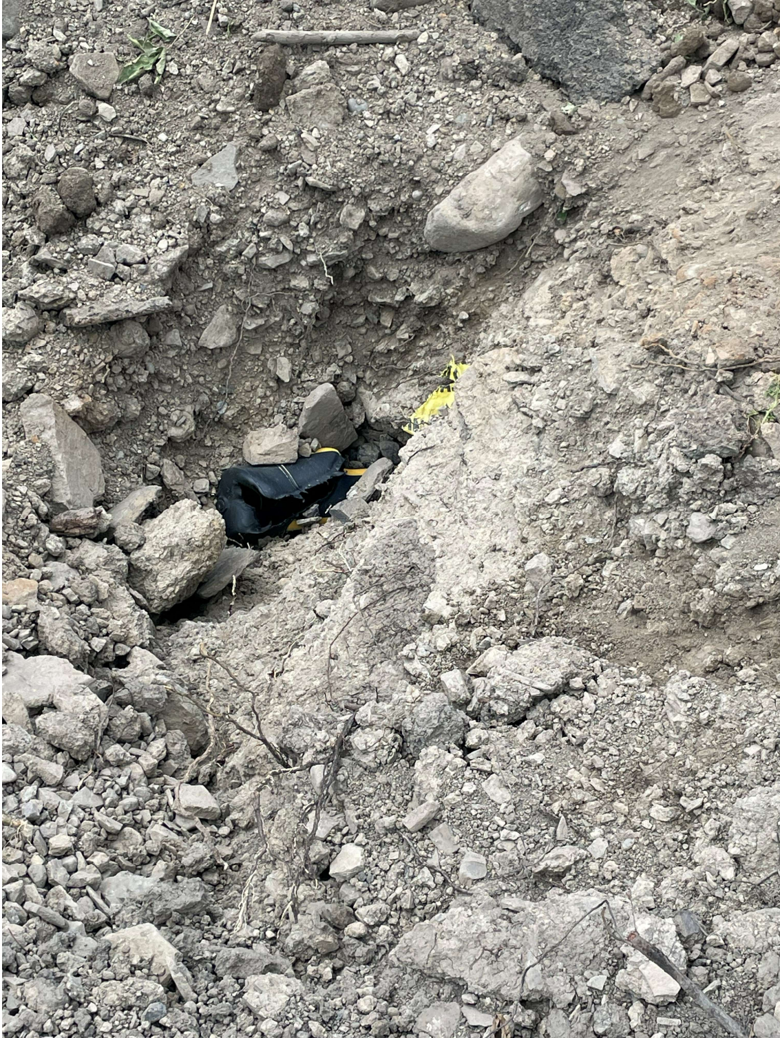
Picture 5: Close up of damaged pipe.
