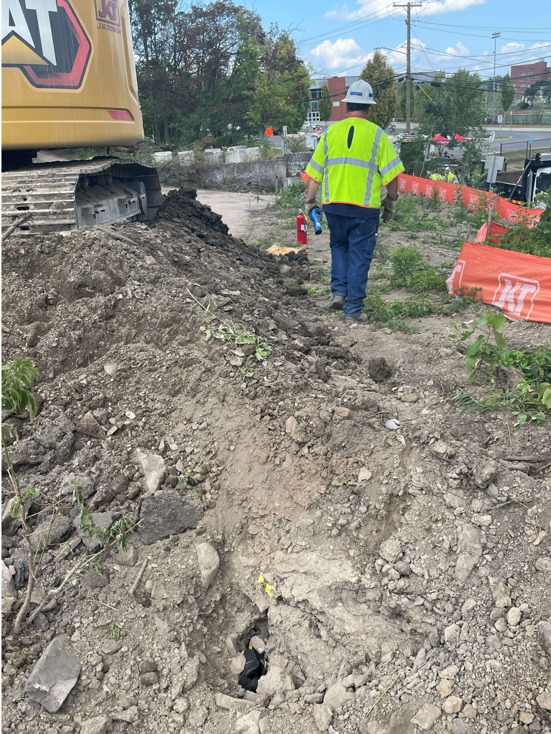
Picture 4: Damaged pipe shown in the hole.
