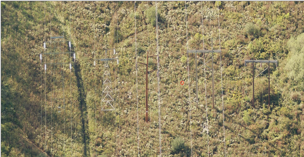
(Left-Right: Existing Lines 114 & 113, Existing Line 112, Existing Line 111, Existing Line 107 and Existing Line 108)
