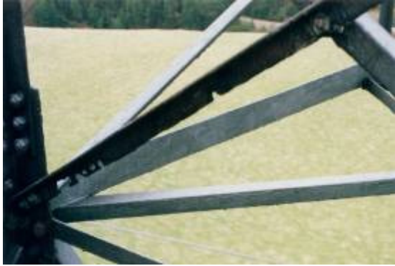
Visual Rating 6 – Very Severe Deterioration Perforated Element – severe physical damage
