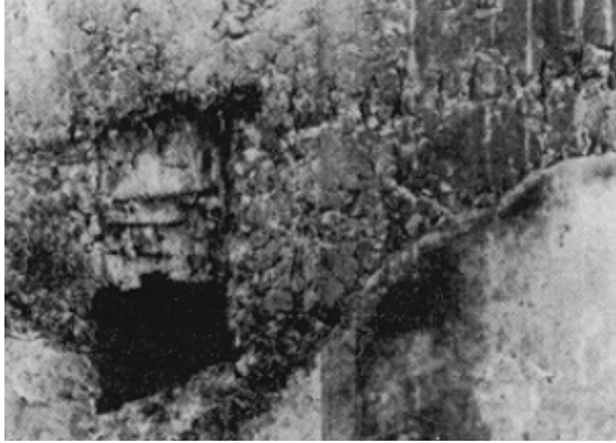
Honeycombing Construction faults, poor workmanship
