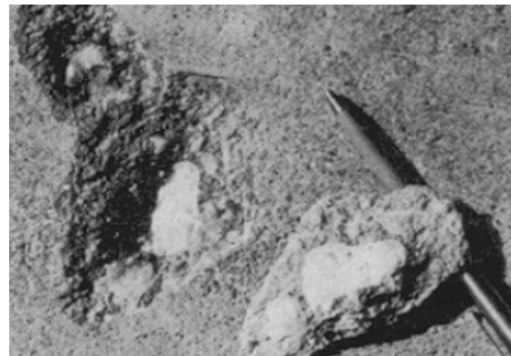
Spalling Development of fragments
