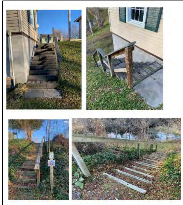
Figure 1. Deteriorated exterior stairs at the Cottage Museum (top) and Towpath Trail (bottom) (Photographs by CCA).
