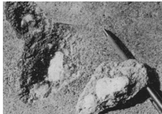
Spalling Development of fragments
