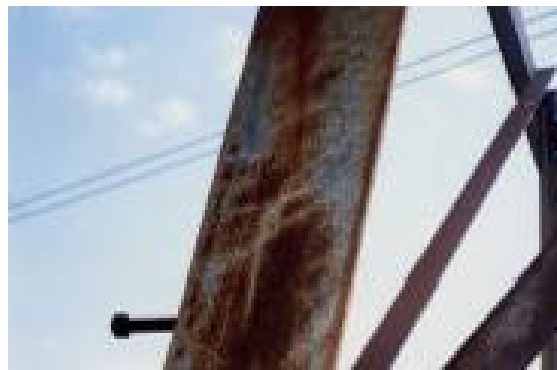
Visual Rating 3 – Light Corrosion Very light surface corrosion, majority of coating intact
