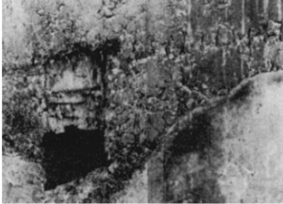
Honeycombing Construction faults, poor workmanship
