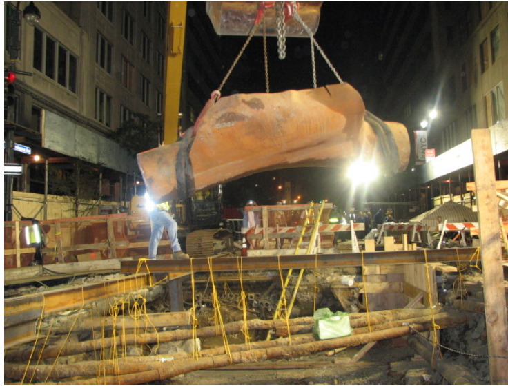
Figure 9 – Photo of Rupture Section Removed from Site
