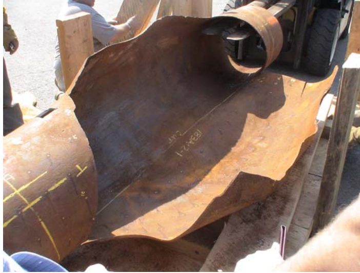
Figure 10 - Photo of Ruptured Steam Main at Astoria Site
