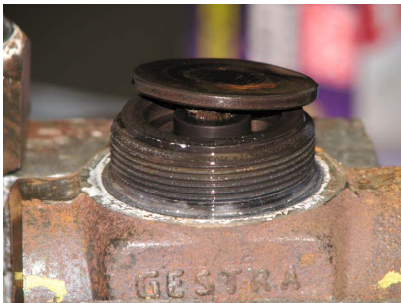
Figure 15 – Photo of Steam Trap (top) With Cap Removed
