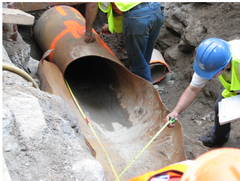
Figure 6 – Photo of Ruptured Main Exposed at Site
