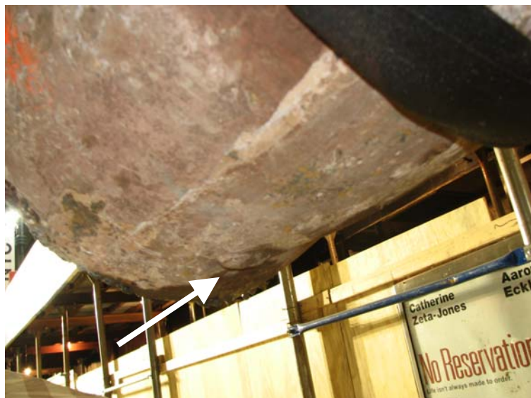
Figure 8 – Photo of Puddle Weld
