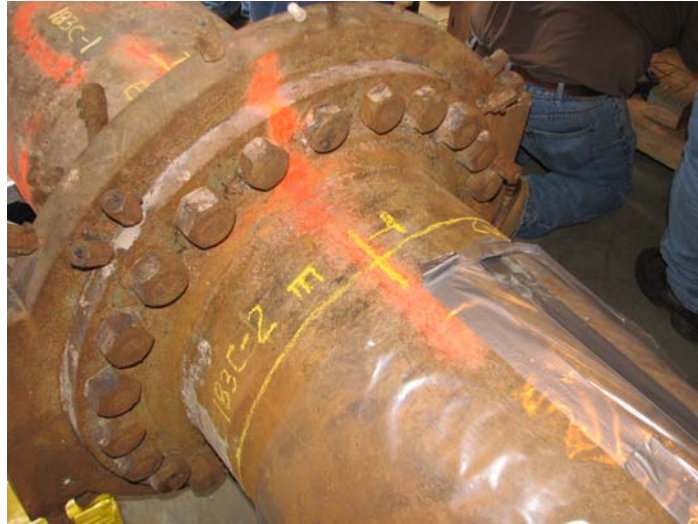
Figure 7 – Photo of Flange with Leak Sealant Injection Clamp
