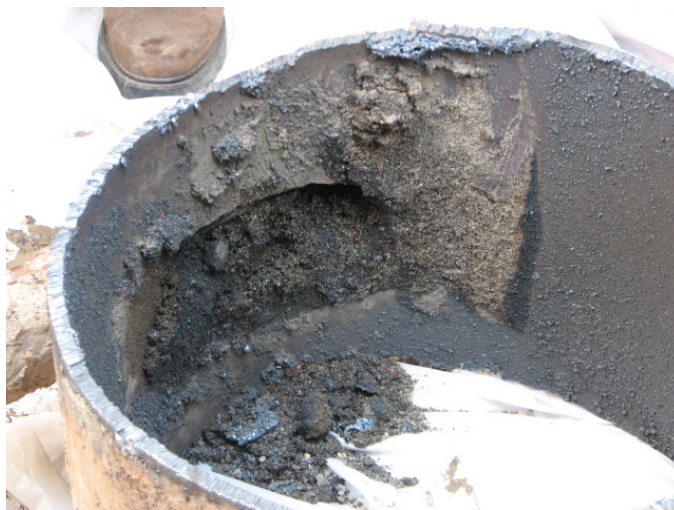
Figure 17 – Photo of Debris in Fish-mouth Connection
