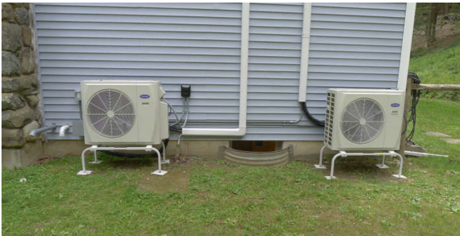
Figure 29: Air Source Heat Pump System Installed at a Central Hudson Customer Residence
