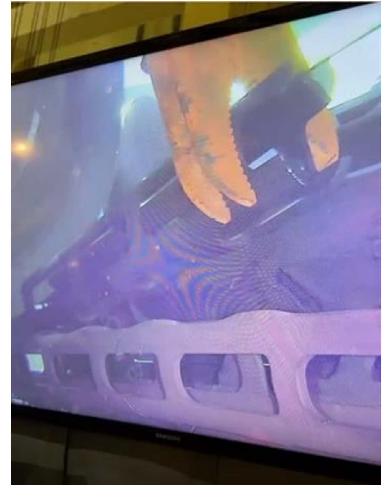
Upper Photos: U2 cavity segmentation use saw and under-water tools for packaging
