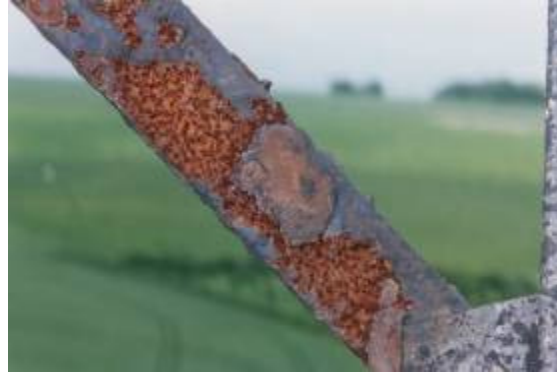
Visual Rating 5 – Significant Pitting Significant pitting – loss of section clearly visible, edges feathered/thinned
