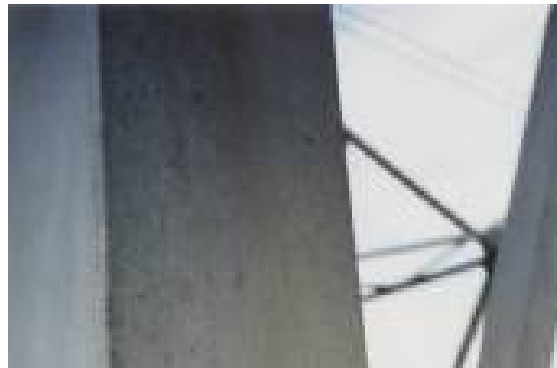
Visual Rating 1 – Serviceable Fully painted – overcoat and undercoat intact Fully galvanized – coating intact
