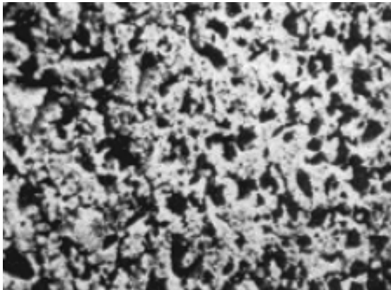
Disintegration Deterioration of concrete into small fragments
