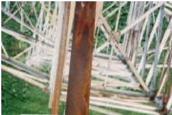
Visual Rating 4 – Light Pitting Some very light edge roughening. Loss of greater majority of coating and zinc layers. Corroded surface would dominate surface preparation – remedial action using wire brush, scraper and brushed paint not sufficient to give greatly increase life
