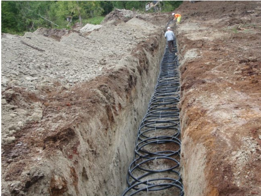
Crews installing the first phase of the Gibsons District Energy Utility. Council decided March 3 to decommission the system. | Island Coastal Economic Trust
