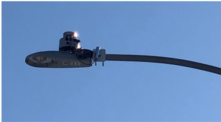
Figure 1. An intelligent streetlight with a NearSky 360™ device and a road surface temperature sensor on an aluminum streetlight pole.
