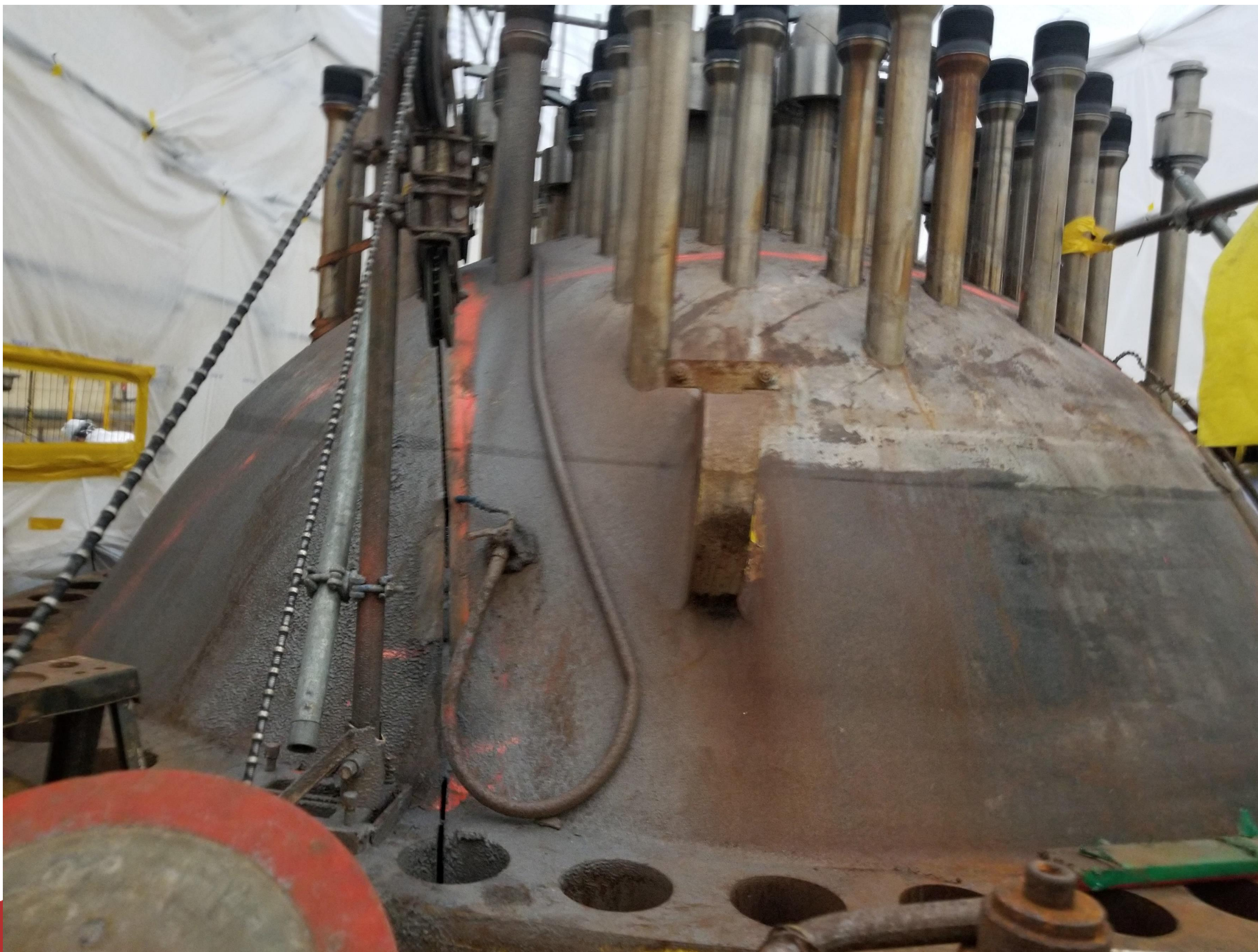
Unit 3 Reactor Head
