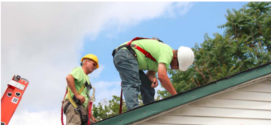
Figure 3-4: Use of safety harnesses by all roof workers is one of several safety protocols followed by the contractor's field installation crews.
