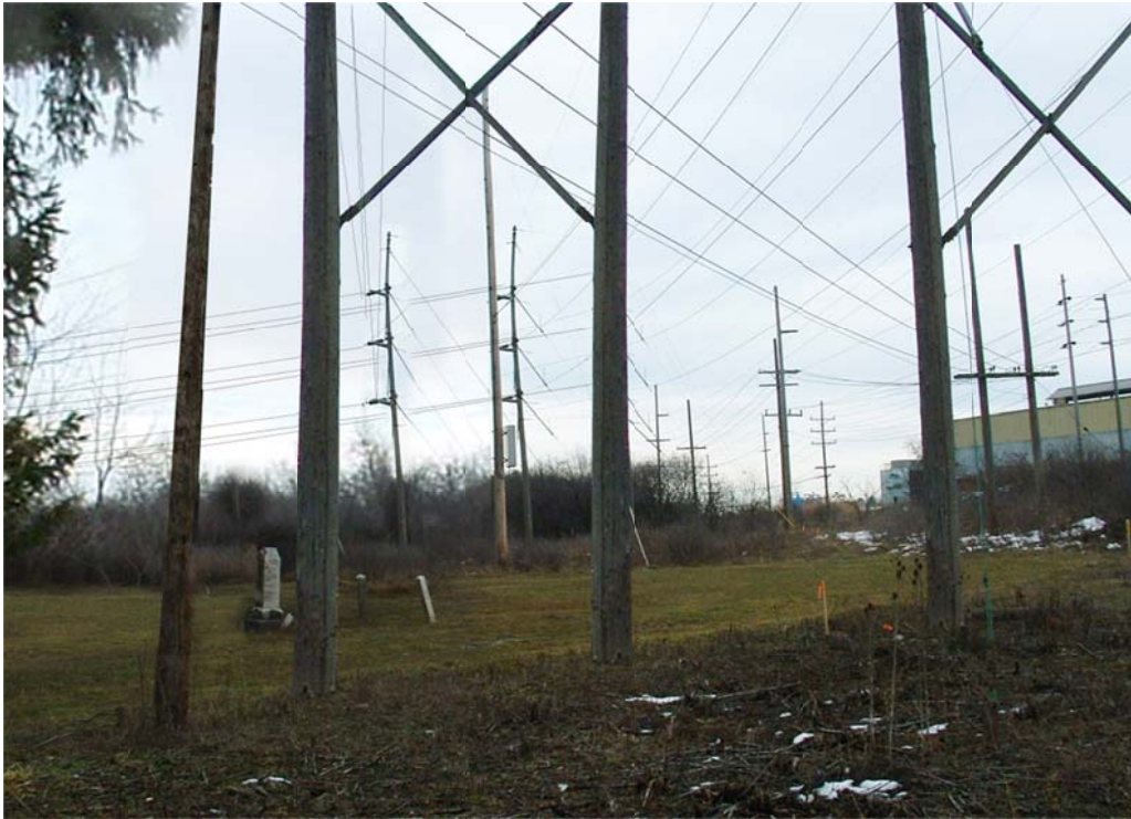
Figure 4-5 Simulation of Proposed Line on Existing NYSEG ROW looking northwest from State Street Substation toward the Cold Springs Cemetery
