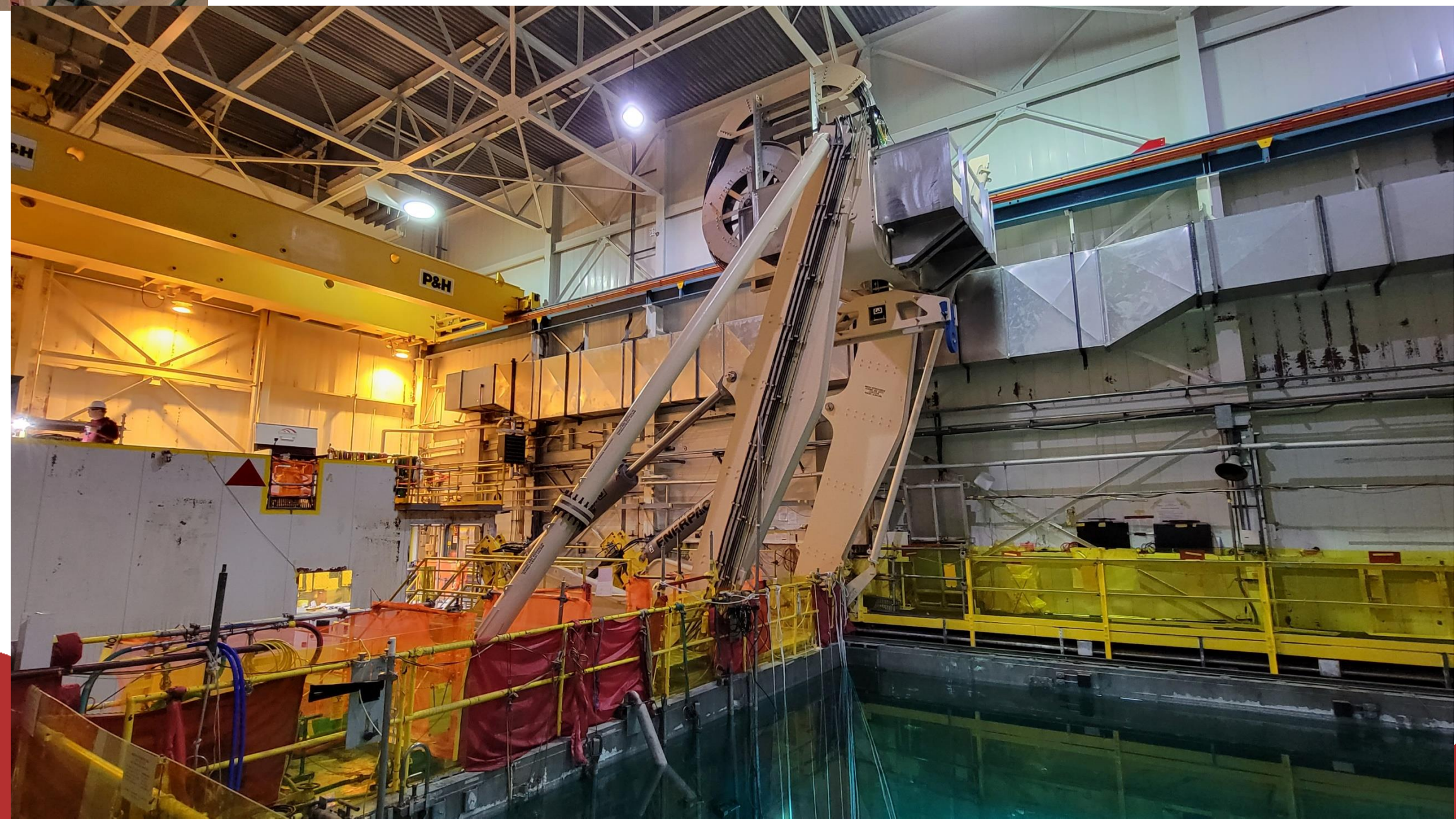
HI-Lift On-Load position over pool
