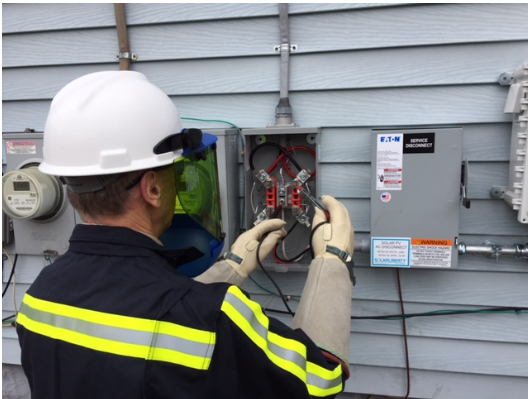
Figure 3-1: Performing a current check prior to installing a dedicated meter on the Solar PV system.
