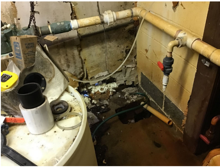
crumbling walls inside treatment building
