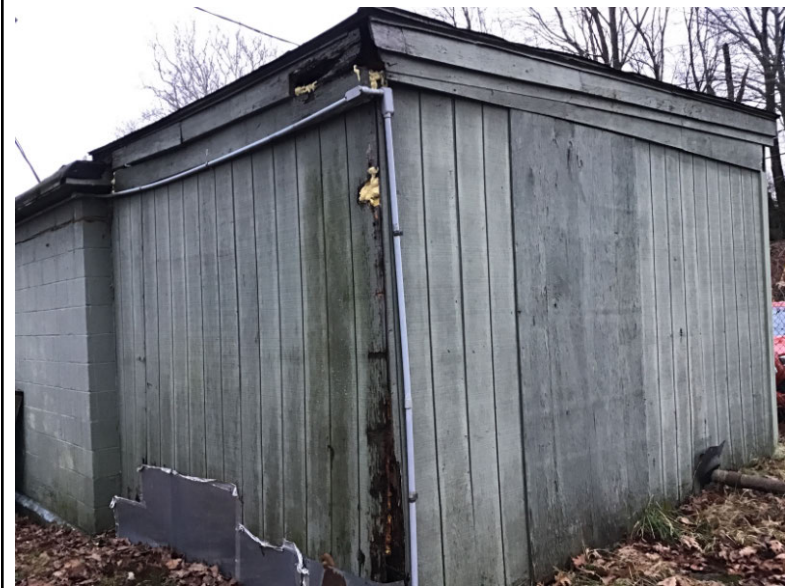
Exterior wall in disrepair, unable to provide vector control. Concerns for structural integrity
