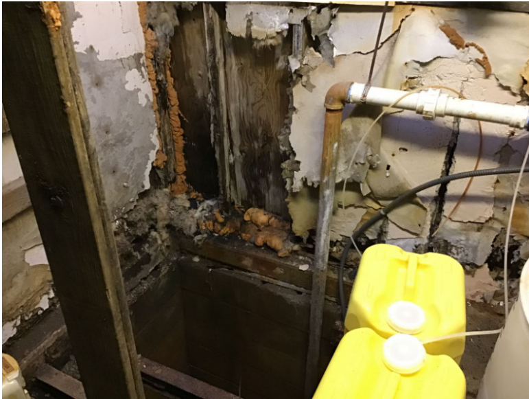
Exterior wall lacking insulation, major damage to structure from weathering
