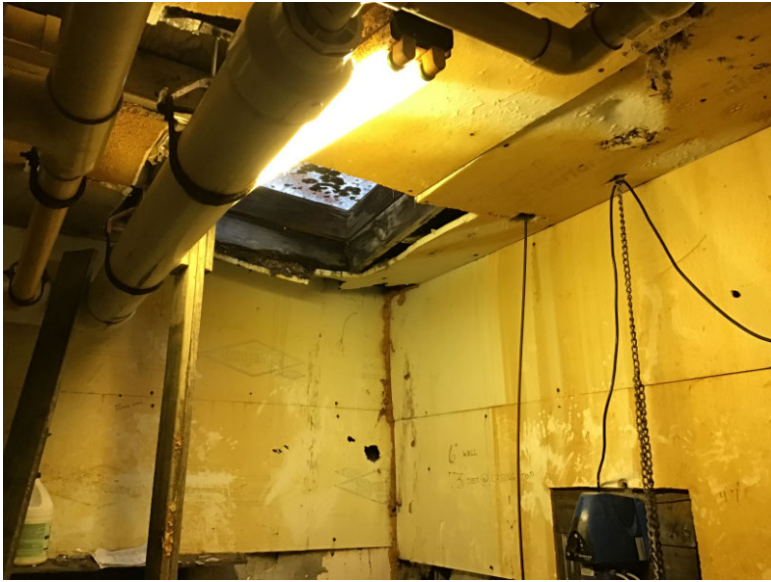
Collapsing ceiling, support beam held up by 2x4s and bottle jack.
