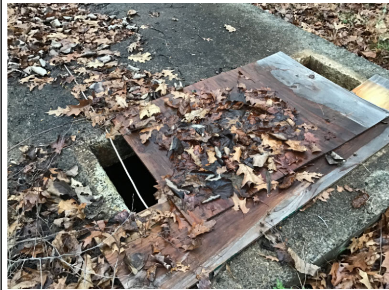
Backwash well pit not properly secured, serious potential for injury or unapproved access
