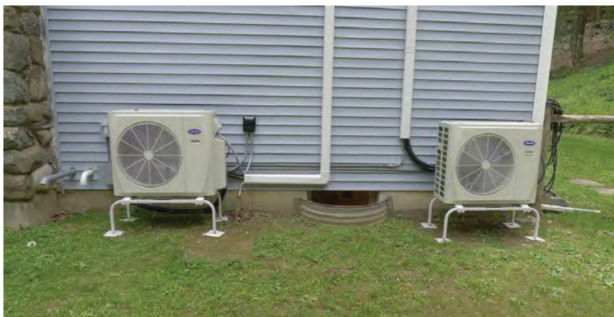
Figure 23: Air Source Heat Pump System Installed at a Central Hudson Customer Residence
