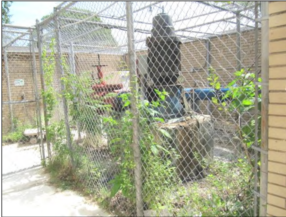
View of Water Pumping Station on East Side of Building to Remain on Property
