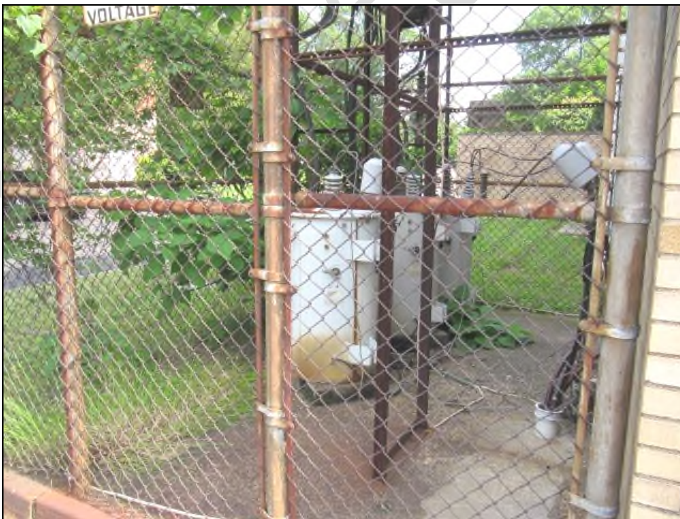
View of LIPA Equipment on West Side of Building to be Relocated from Property
