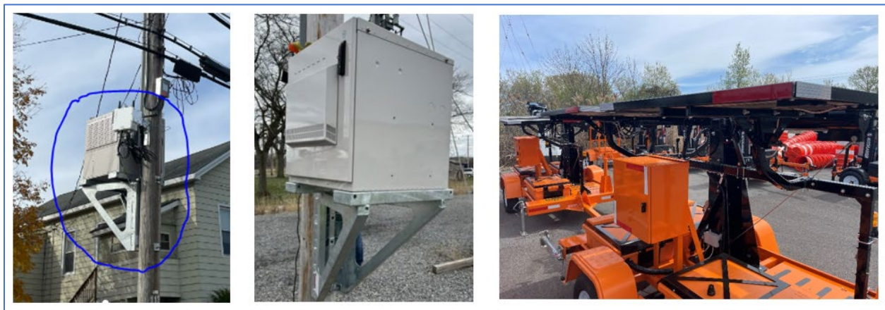
Figure 3.1.2: Pole Mounted extended battery backup solution and mobile connecting grid router
