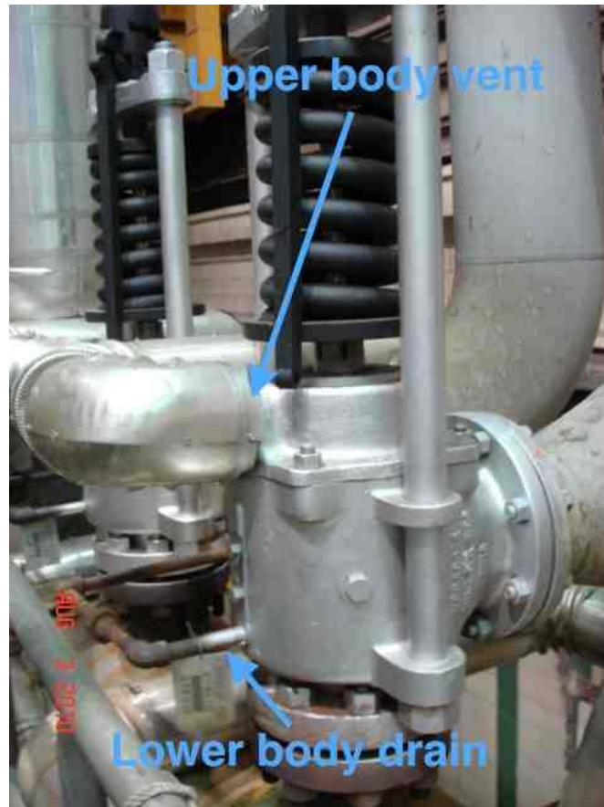
Figure 11– SH safety valve drain/vent connections.
