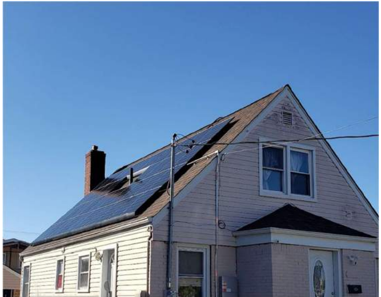
Image 19. Rooftop solar installation. Photo credit: 718 Solar.
