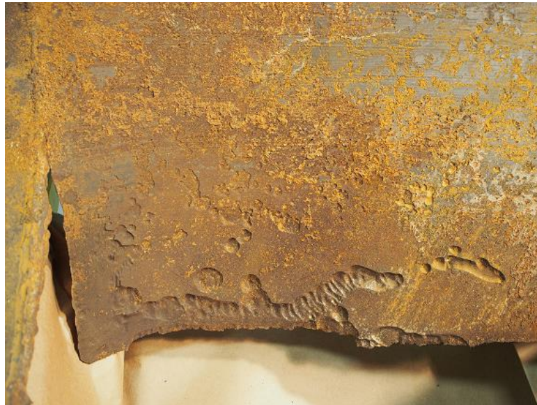
Figure 10 - Flow-Accelerated Corrosion on Bottom of Pipe, Taken by Affiliated
