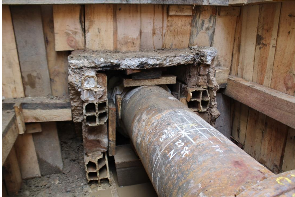
Figure 3 - Photo of Steam Main in Older-Style Housing along Fifth Avenue, between 20th Street and 21st Street. Taken by Staff
