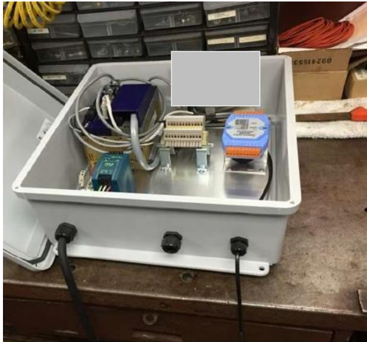
Figure 16 - Photo of Remote Telemetry Unit (RTU) Box
