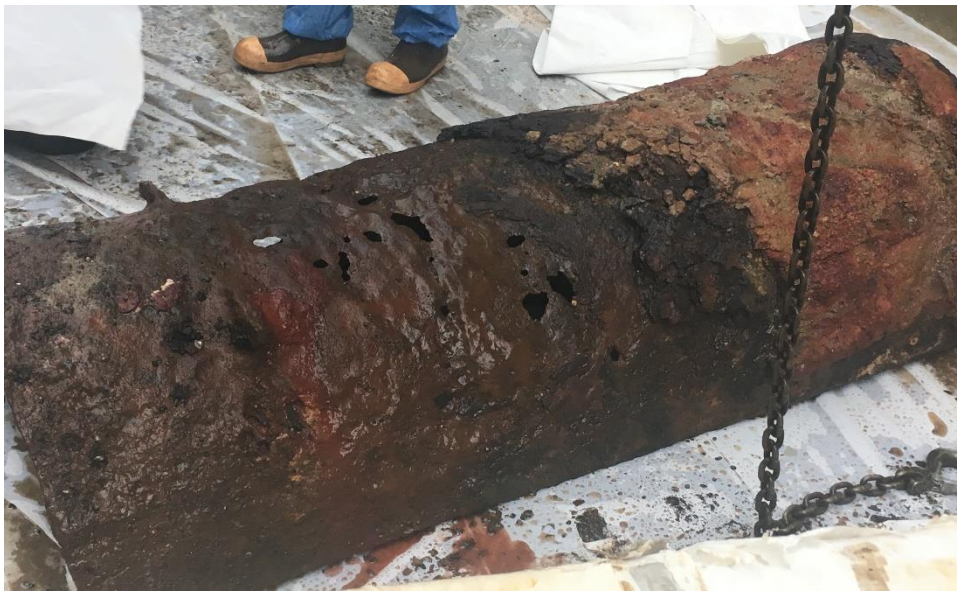
Figure 11 - Cast Iron Housing Removed from Rupture Site, Image Taken by Staff
