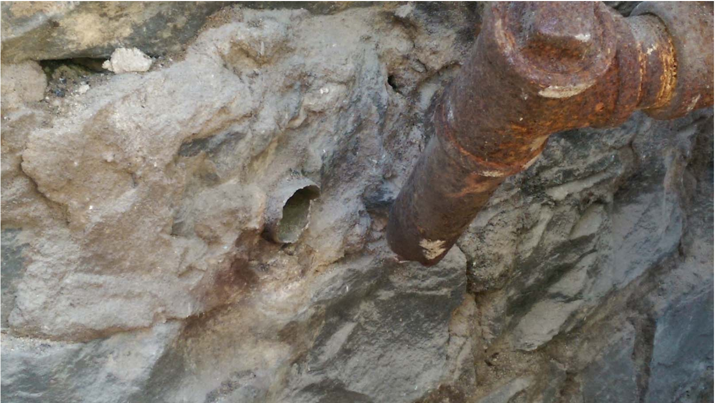
Photo 9 (8/11/2014) - 1 ¼ inch steel service pipe where it was sheared off at the foundation wall.
