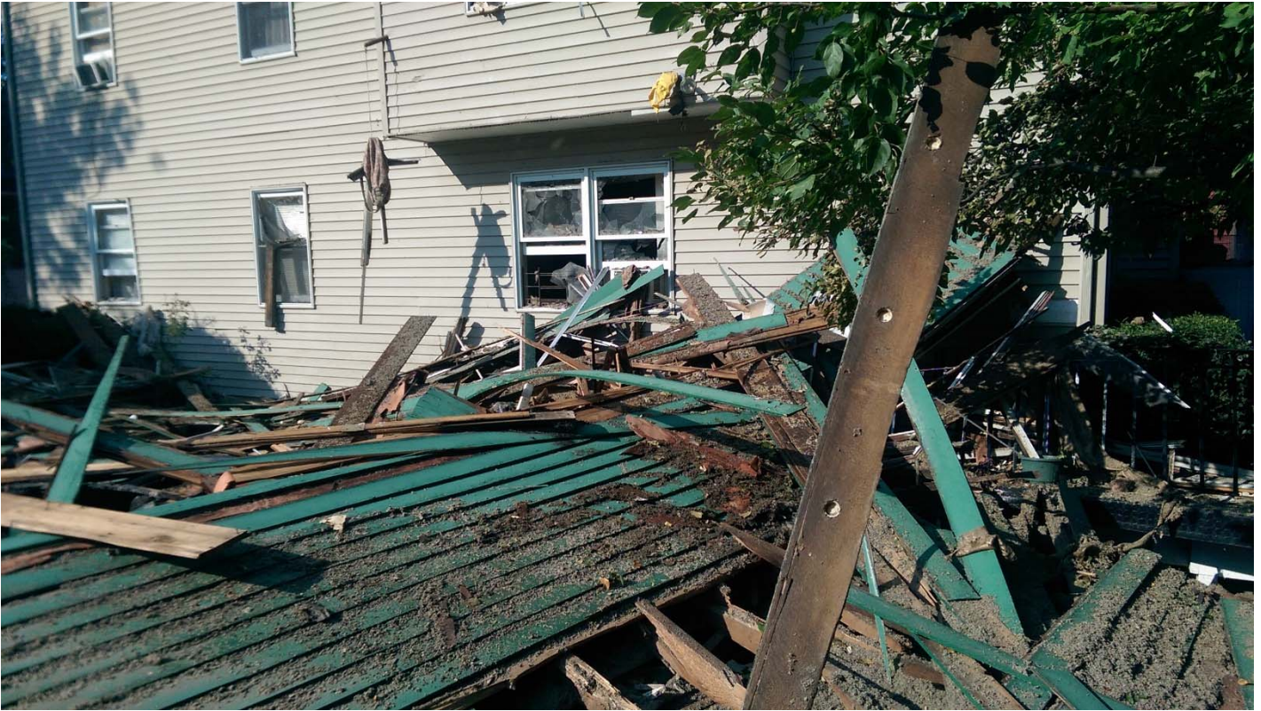
Photo 3 (8/10/2014) - 304 Paige Street exterior damage.
