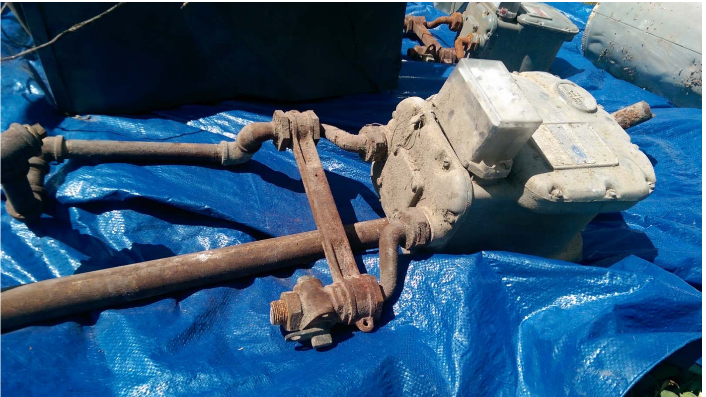
Photo 10 (8/11/2014) – First floor inside meter and service valve in “on” position.
