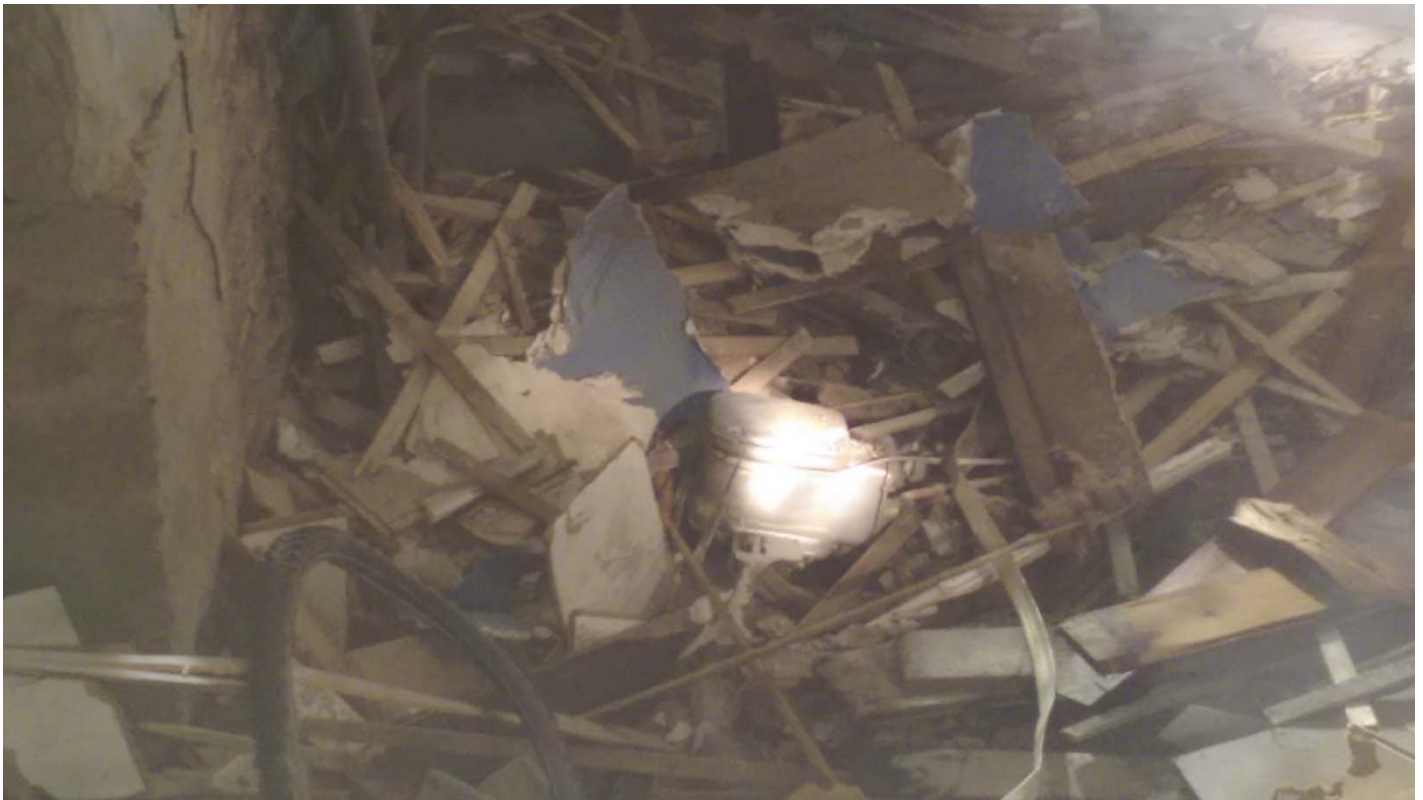
Photo 6 (8/11/14) - A gas meter on the floor of the basement, before it was moved for observation.
