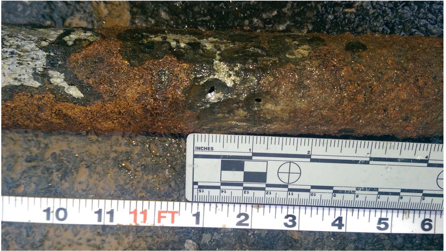
Photo 15 (8/12/14) - The pinholes found in the 1 ¼ inch service line.
