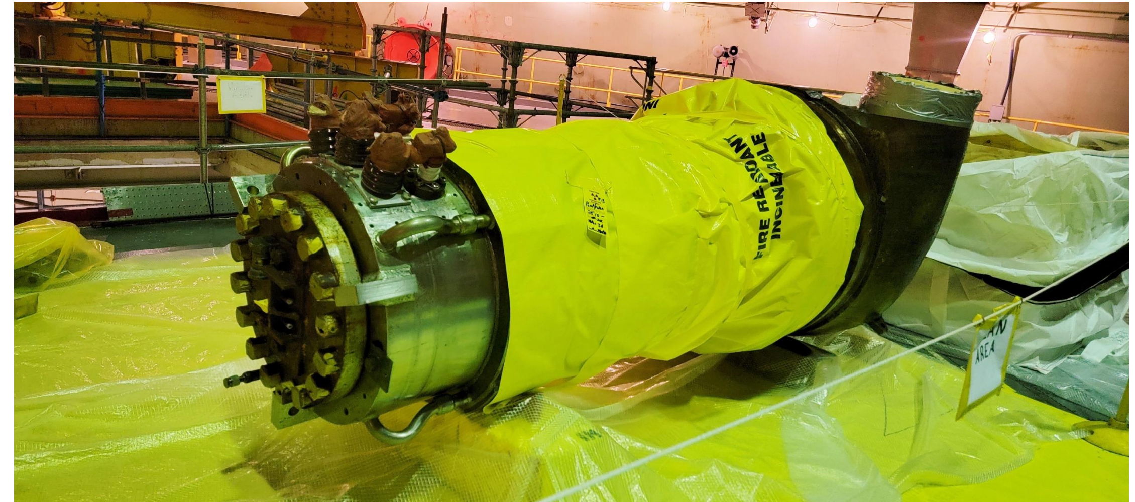
Unit 1 Reactor Coolant Pump
