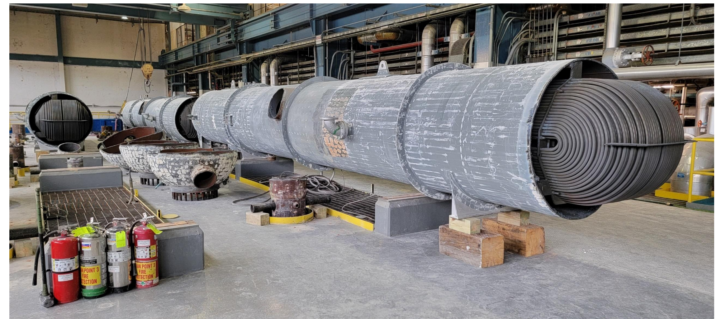
Unit 3 Feedwater Heater
