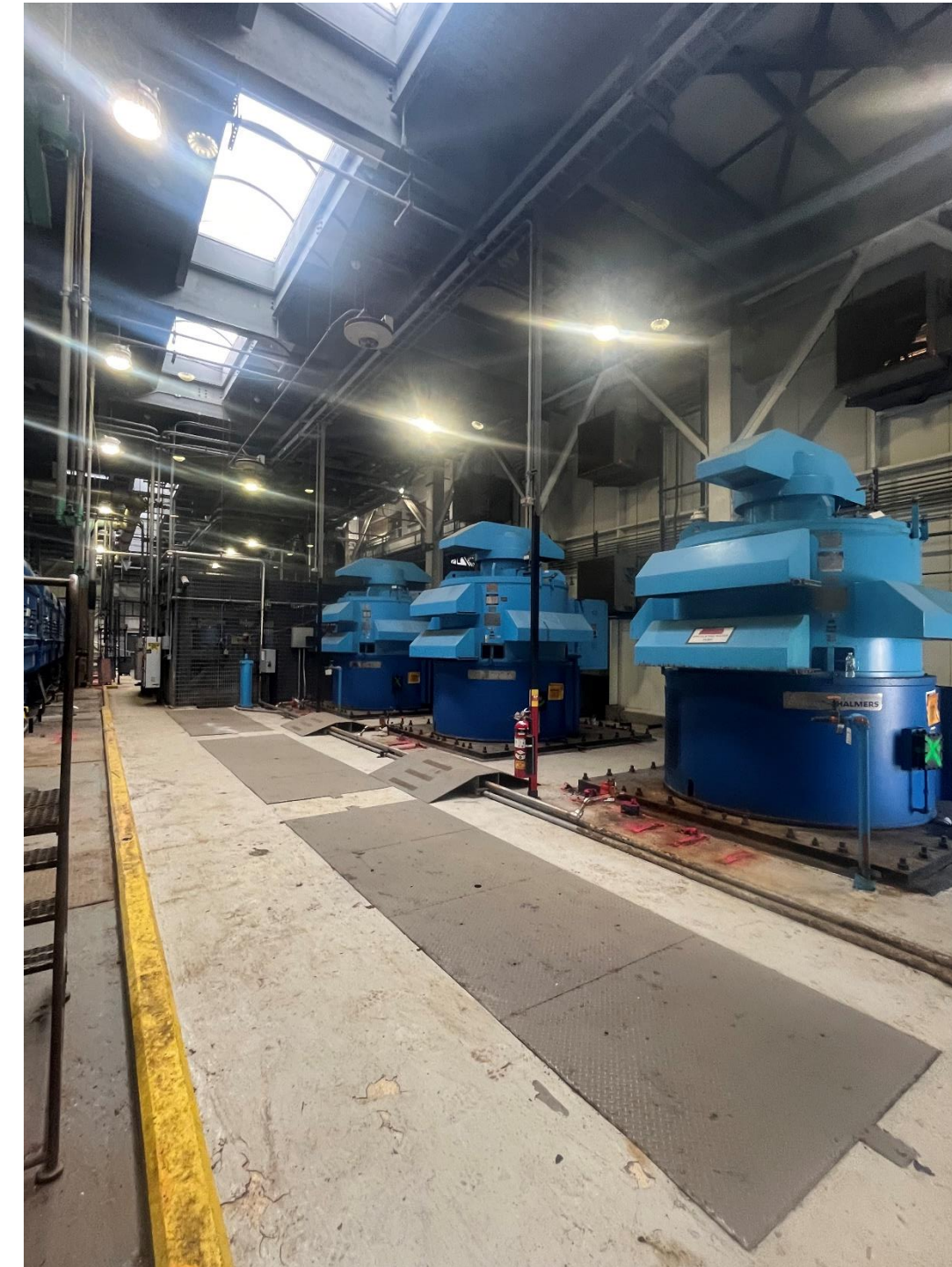
Unit 3 Circulating Water Pumps
