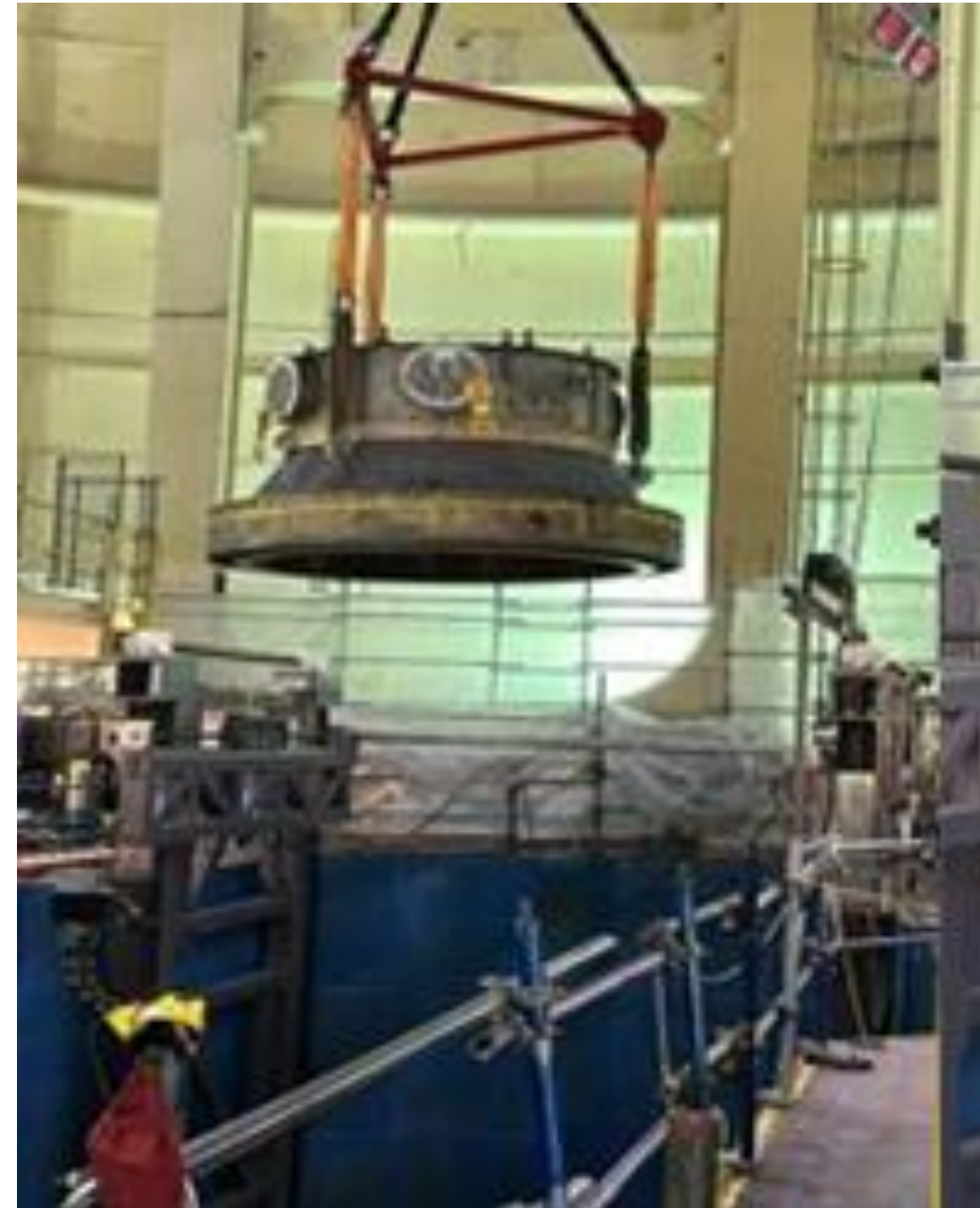
Unit 2 Reactor Head
