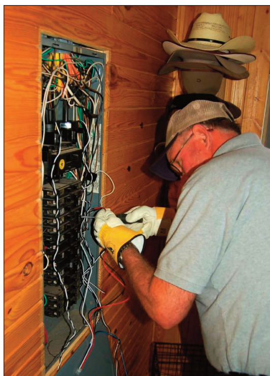
FIGURE 3. Sub-metering equipment installation in participating home. Source: www.wfec.com/media-center/photo-galleries/geo-validation-underway
