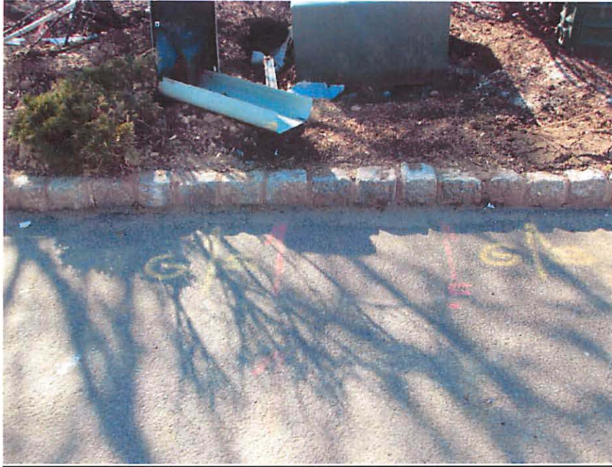
Image #6 – Service Line Mark-Outs at Transformer Placed by ORU – Taken by Arpit Mehta
