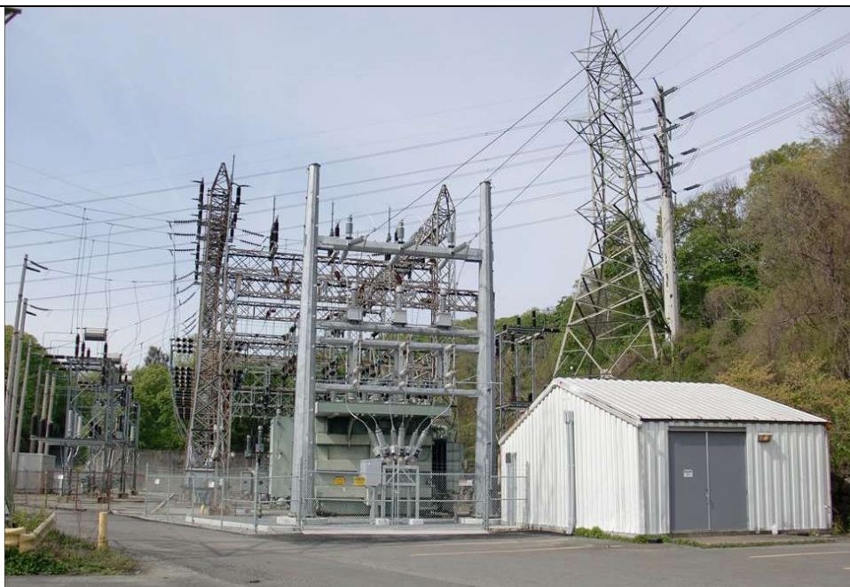
Figure 1. View of the Lovett 138kV substation yard with the control house located in the foreground to the right (white building).
