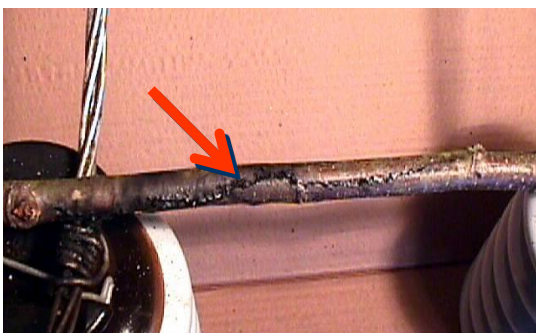
Figure H4. A completed carbon path, fault occurred
