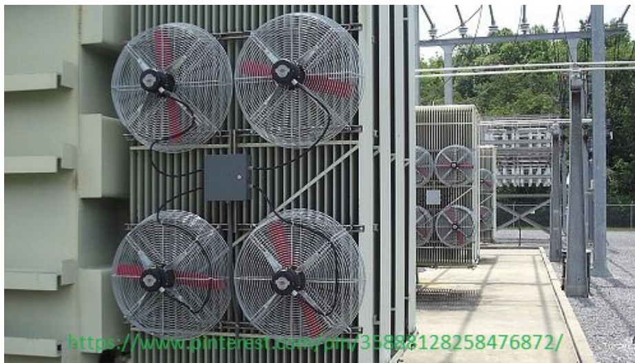
Figure 1: Transformer cooling using external fans.
