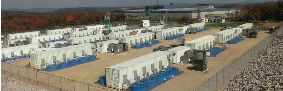
Photo 20: 20 MW Flywheel Storage, Hazle Township, PA (Photo Credit -Beacon Power Website)
