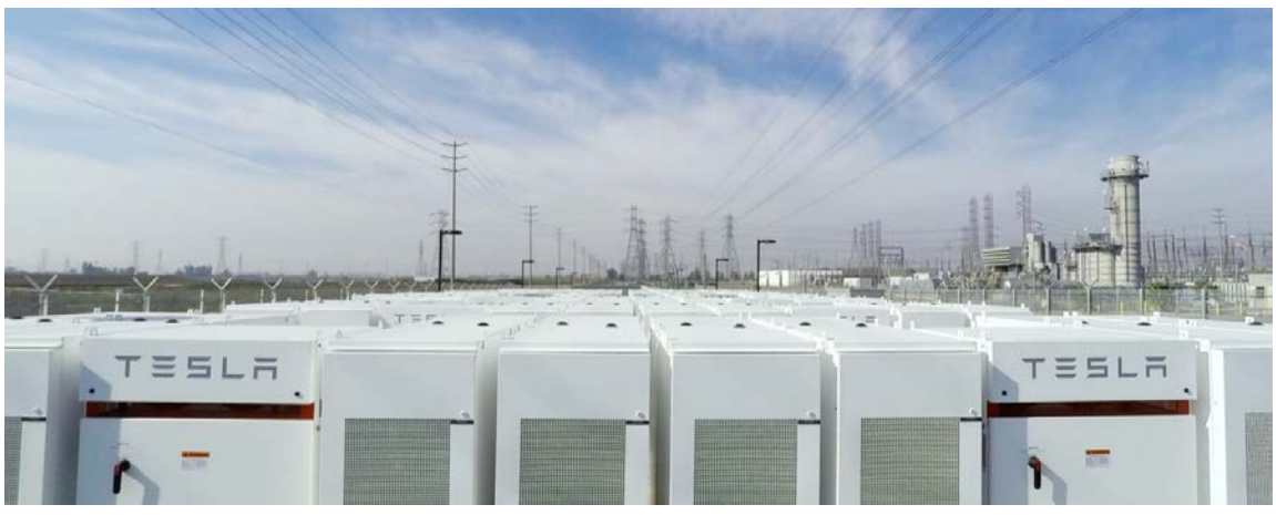
Photo 19: 20 MW/80 MWh Battery Storage - Southern California Edison (Photo Credit, Tesla website)
