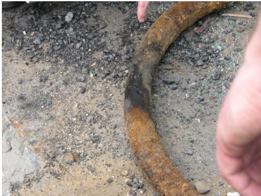
Photo 3 - Hole in electric conduit
