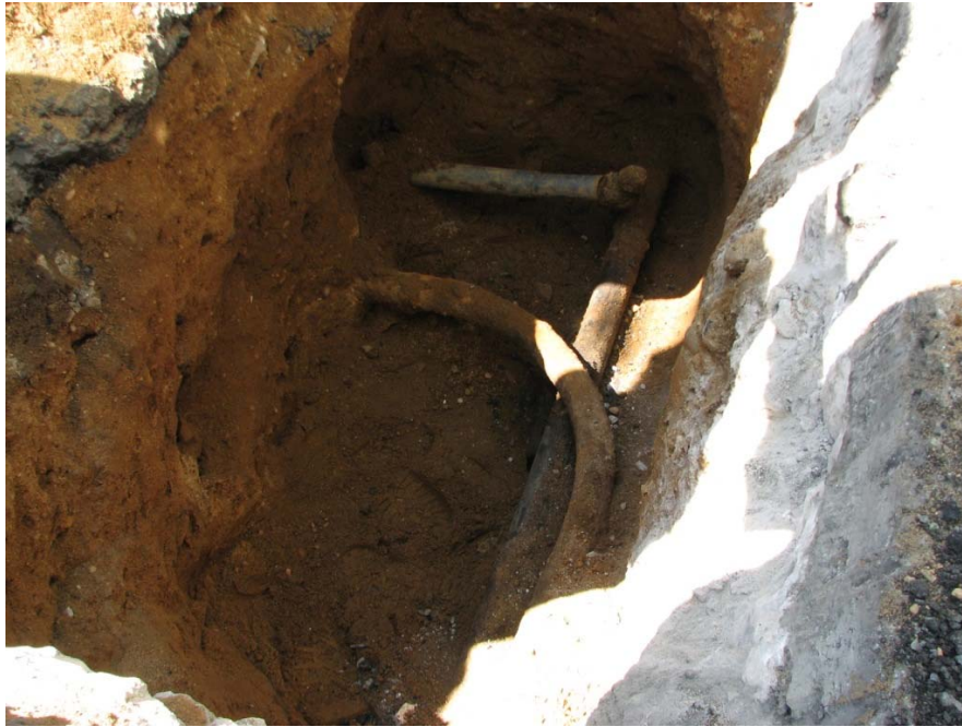
Photo 1 - Electric conduit in contact w/gas main
