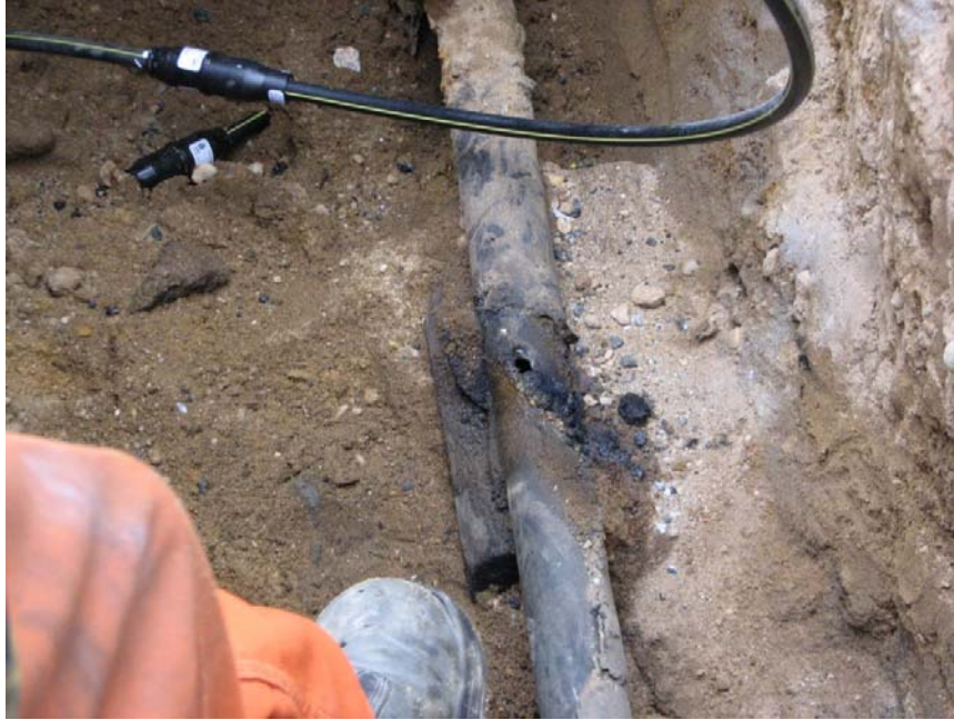
Photo 2 - Hole in the gas main
