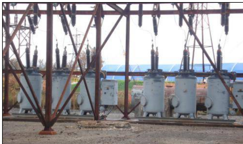
Photo II-5 Deteriorated Rome Station Structures and Foundations
