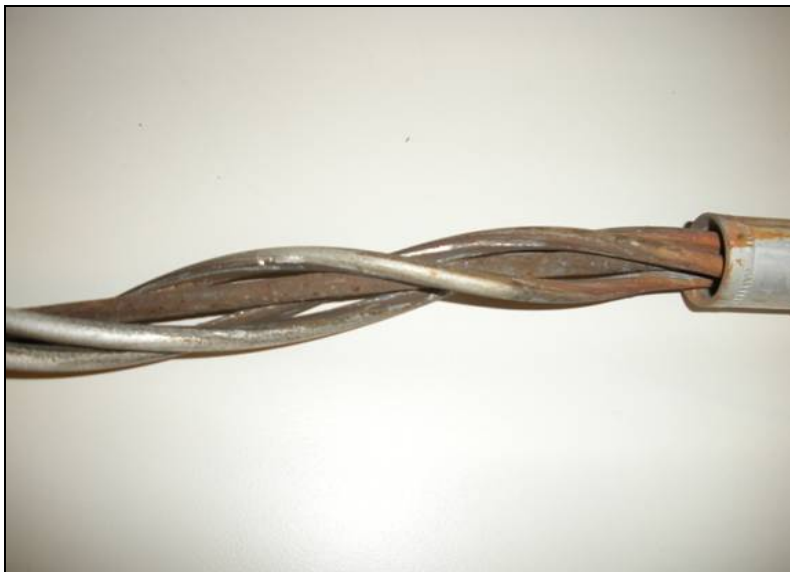
Photo II-2 Early onset of Corrosion
