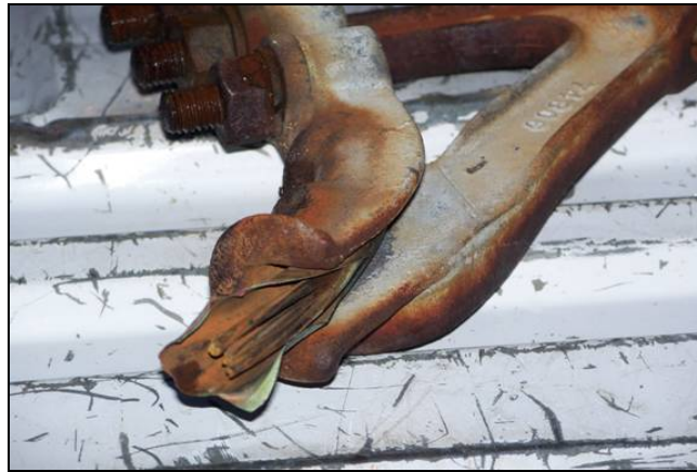
Photo II-3 Clamp Failure on Ticonderoga – Whitehall #3 Shield Wire
