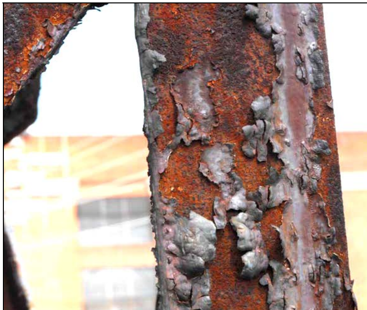
Photo II-7 Deteriorated Steel Structures at Lockport
