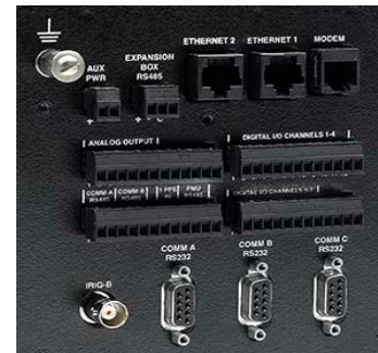
Switchboard Meter Rear View
