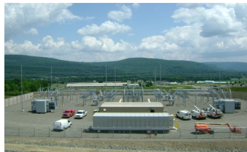
Sullivan Park Substation
