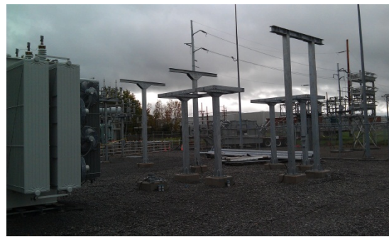
115 kV support structures
