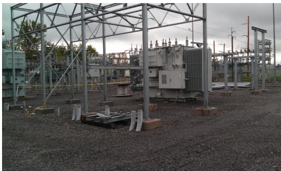
Transformer & vacant distribution bays
