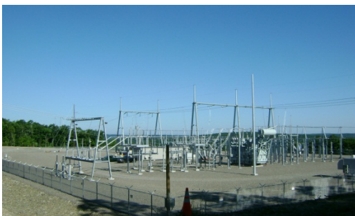
Stoney Ridge Substation
