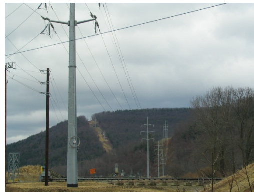
Typical Steel Transmission Line
