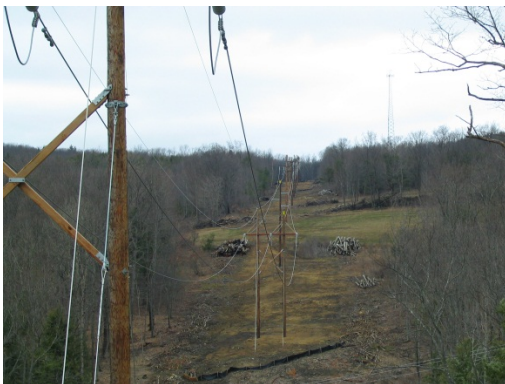
Typical Wood Transmission Line
