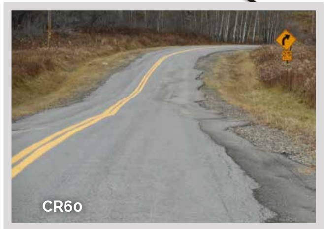
County Road 60, 7% uphill grade and major washout issues. Logisticus does NOT recommend to use this road
