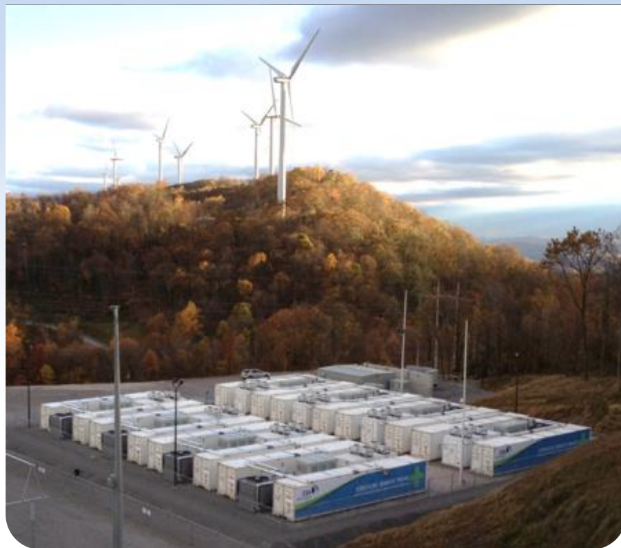
64 MW AES Laurel Mountain Battery Array Competitively bid into PJM Interconnection
