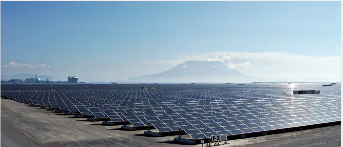
Photovoltaics in Japan: SMA Sunny Central CP JP inverters are in operation in the Kagoshima PV power plant and in densely populated areas of the island country.
