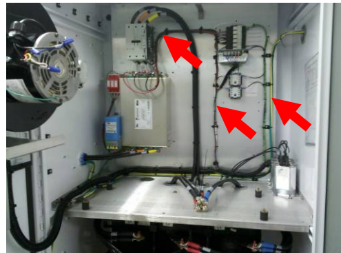
Controlled Wire Routing
