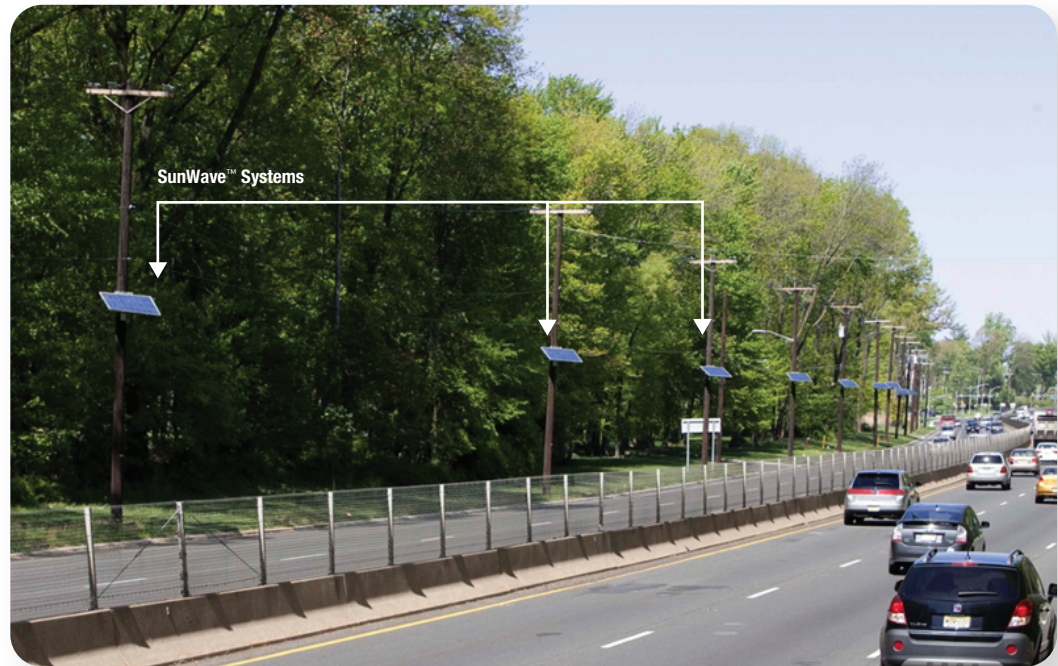
Fig. 1 Petra Solar's "highly distributed" SunWave™ pole mounted PV power generation system
