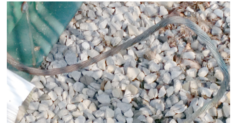
Copper ground wire thefts at substations have spiked since Aug. 1, especially on the east side of the Hudson River. The thefts create potential safety hazards for employees who enter substations.
