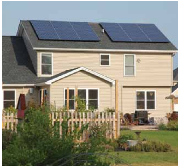
6.9 kW PV System, Lancaster, NY
