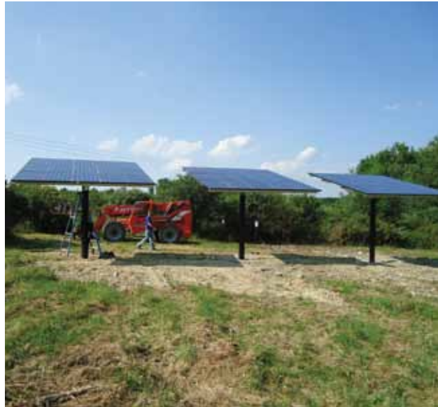
11.025 kW PV System, Ithaca, NY
