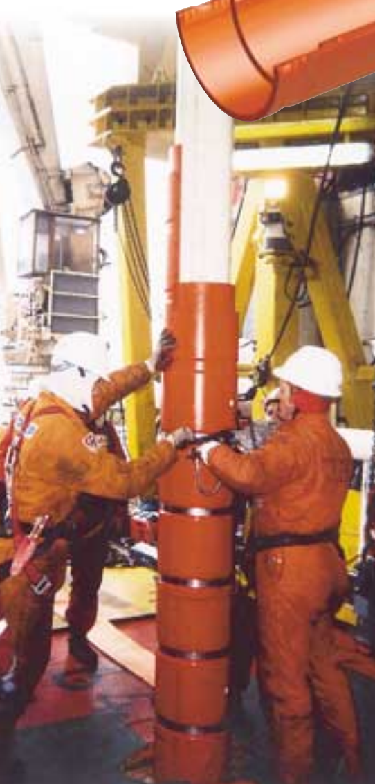
Touchdown protection on to a flexible riser for BP Schiehallion.
