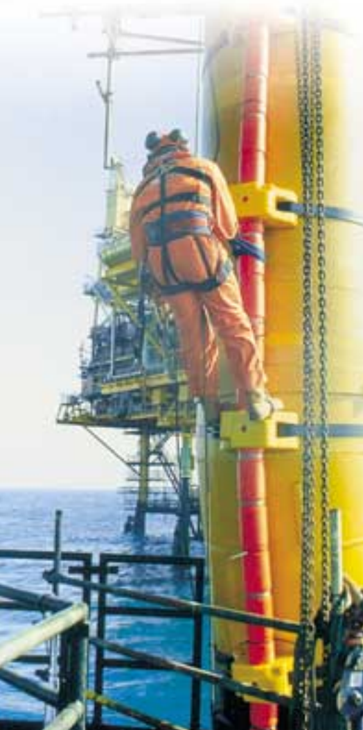
Installation of CRP's Uraduct® retrofit riser system on Shell Leman BH Platform in the North Sea
