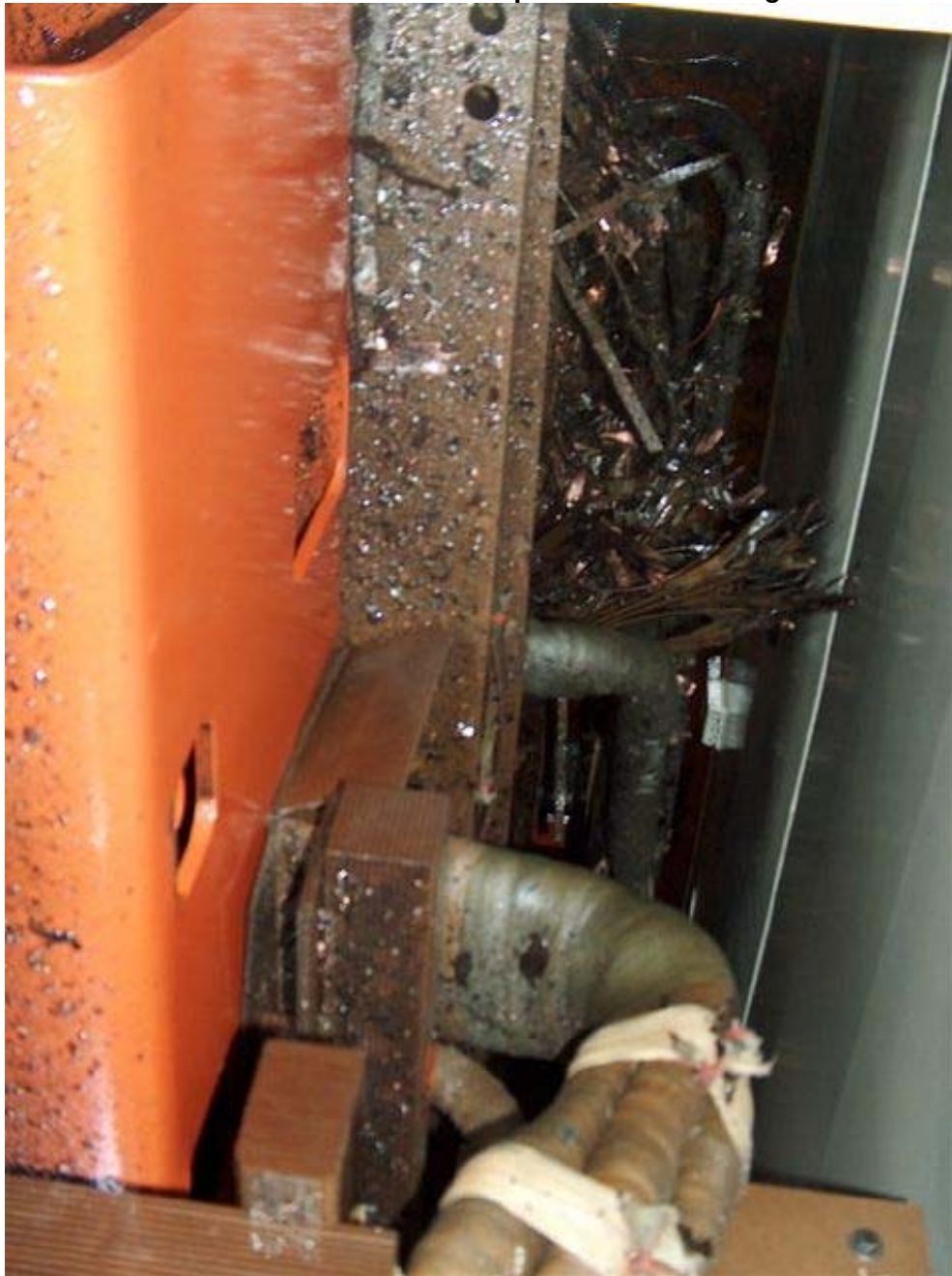
Bethlehem LTC Transformer 2: phase 3 HV winding failure
