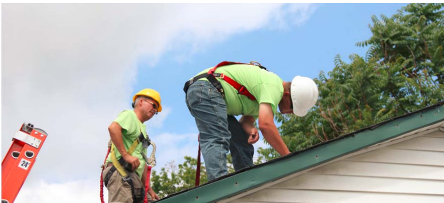
Figure 3-4: Use of safety harnesses by all roof workers is one of several safety protocols followed by the contractor's field installation crews.
