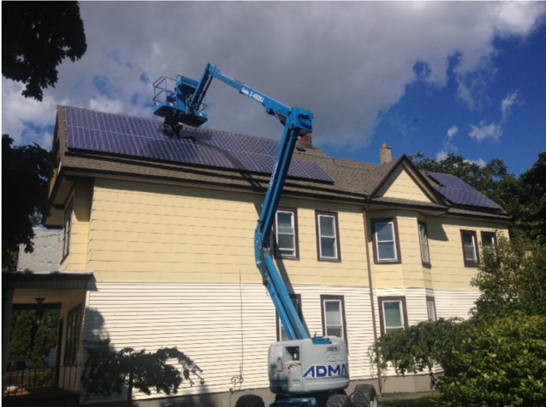
Figure 3-2: Installing the second rooftop solar PV system in the Fruit Belt neighborhood.
